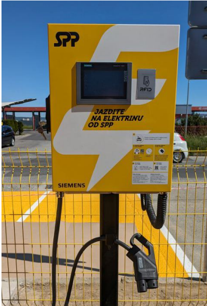
DC 30 kW charger
